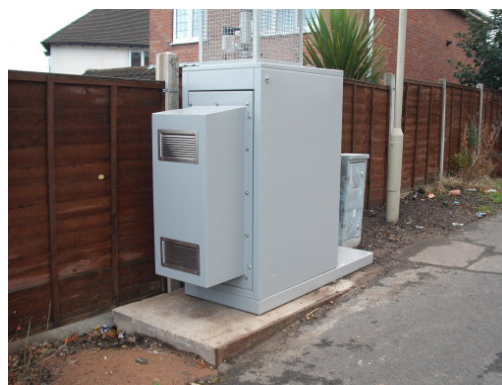
Air Quality Monitoring Station at Burnt Tree Island, Dudley
