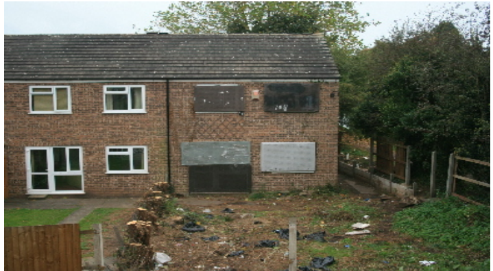
The vandalised house at Essington Close
